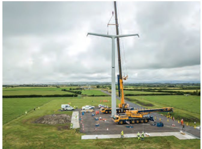
Standing at 35 m in height, the new pylon design forms a 'T' shape and is about one-third shorter than the traditional lattice pylon design.
