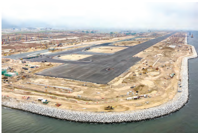
ABOVE AND BELOW: Pavement works for the new third runway were completed in June 2021. It is scheduled for commissioning in 2022.
