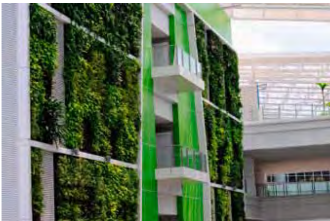
Green wall at Block C
