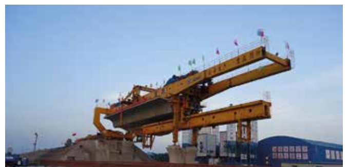
XCMG equipment helping to lay the first box girder for the inter-city railway between Qingdao city and Rongcheng city.
