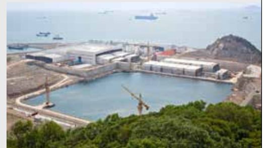
The 180 m long tunnel tube sections are pushed from the field factory into a dry dock, sealed by means of bulkheads, flooded and then towed to their final positions.
