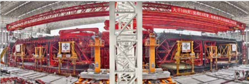
Two hydraulically-operated shuttering machines are being used for the efficient realization of 33 tunnel elements with a length of 180 m using the incremental launching method.
