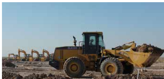
An XCMG wheel loader working on the Siwera Sewage Treatment Plant Project in Iraq.
