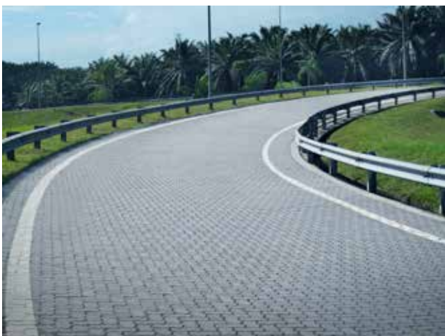
Product: ICP Product profile: Sunpave Thickness: 80 mm Size: 223mm X 111mm Location: SILK Highway, Kajang, Selangor, Malaysia.
