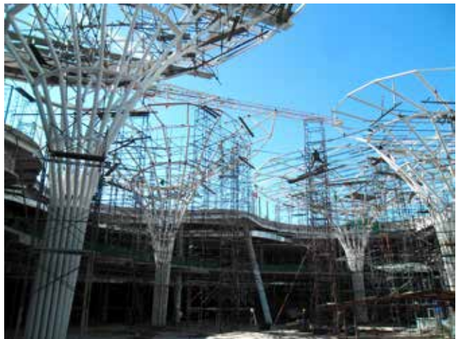
Each of the eleven umbrella structures includes an estimated 300 steel tubes, all of which must fit precisely together.
