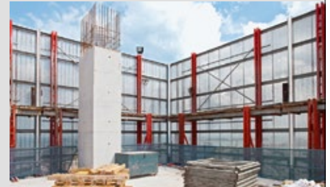
With the PERI RCS Rail Climbing Safety Screen, the slab edges on the upper floors are completely enclosed.
