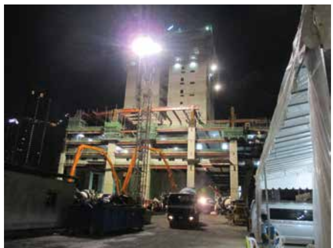
A total of 42 hours taken to complete the foundation between 1.00pm on 3 May 2014 to 7.00am on 5 May 2014. Photo: © GuocoLand
