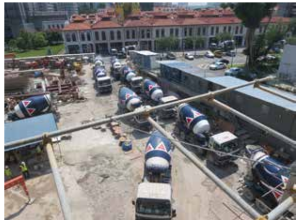
103 trucks taking an average of 14 trips each, making a total of 1,489 truck-trips. Photo: © GuocoLand
