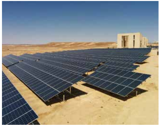
The 1.028MWp solar photovoltaic plant at the Ma’an Development Area in the Hashemite Kingdom of Jordan. Photo: © Phoenix Solar Pte Ltd
