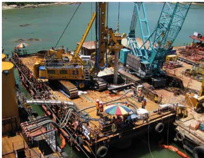
Bauer is involved in the HK-Zhuhai-Macao Bridge project, currently under construction on the Pearl River Delta.
