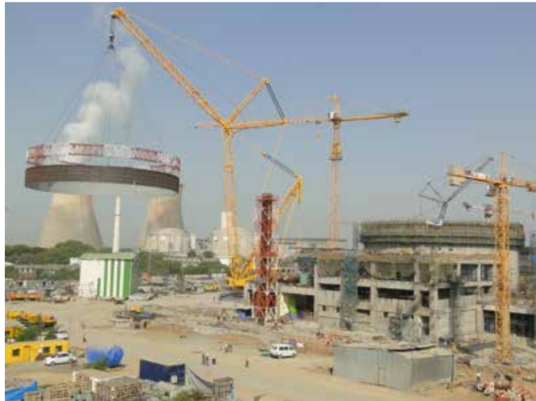
A Liebherr LR 11350 lifts a complete pre-formed ring liner during the construction of reactor block 3 at the Kakrapar Nuclear Power Plant.
