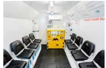
Inside a MineARC refuge chamber.
