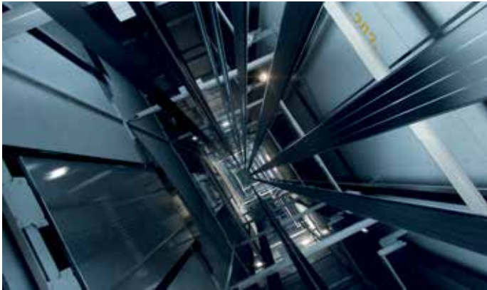
KONE UltraRope in elevator shaft. Photo: © KONE
