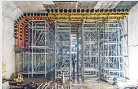
PERI UP Rosett Flex in combination with ST 100 Stacking Towers and the VARIO GT 24 Wall Formwork system.
