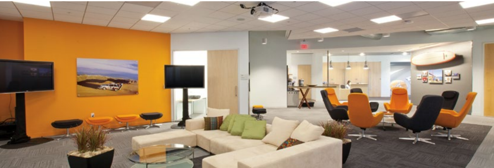
Redwood intelligent lighting network solution is deployed in this office space
