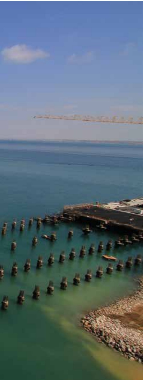
Above: Construction work on the container terminal of the Paita Port in Peru is in full swing.
