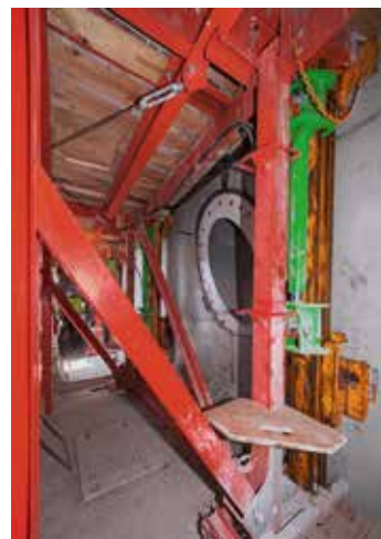
Above: The two A-shaped inclined bridge pylons steadily rise up into the air with the Peri ACS climbing formwork system finally reaching a height of over 300 m.
