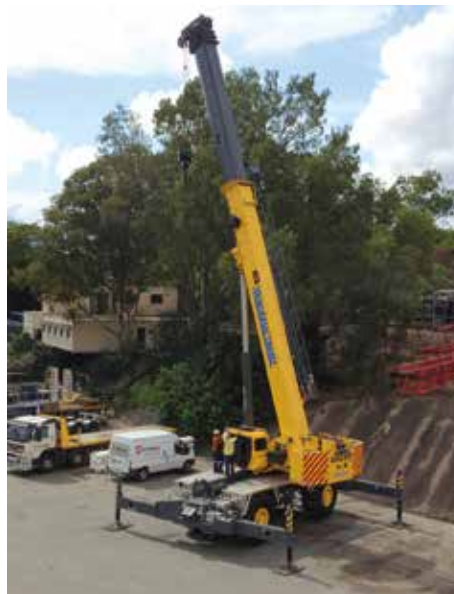
Left and below: The Grove RT9130E-2 cranes are currently working on the Ichthys LNG project. They are used almost all day, every day to keep the project on its ambitious schedule.
