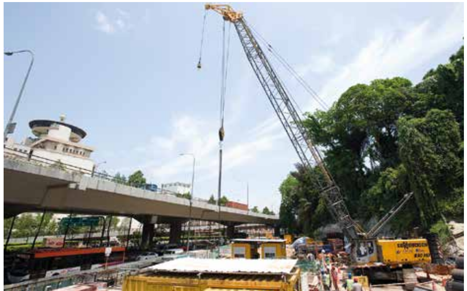
A Sennebogen 690 HD at the construction of Sentosa Gateway Tunnel in Singapore.
