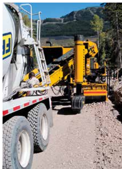
Above and left: Bears paw Contracting uses a Gomaco Commander III to slipform both curb and gutter and monolithic sidewalk with curb and gutter on the new Whiskey Jack subdivision in Sparwood, Canada.
