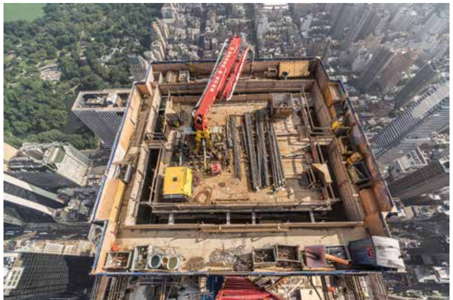
Top: The building core is moving along thanks to the SCP Super Climber, the automatic climbing formwork custom-made for the US market.
