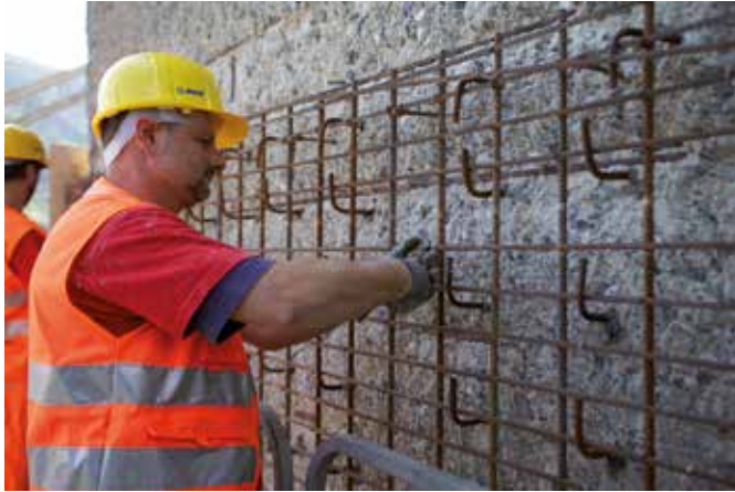
Placing the new reinforcement on the surface after removing the deteriorated concrete by hydro-demolition.
