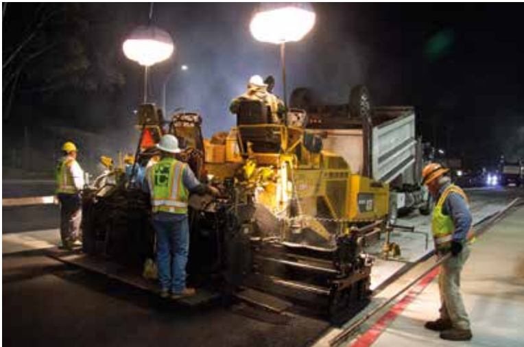
Left: Paving widths were usually 5.5 m though the contractor sometimes utilised Cat's wing extensions to achieve a width of 6 m.
