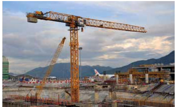
Two Liebherr 380 EC-B 16 Litronic flat-top cranes are working on the expansion of Hong Kong International Airport.
