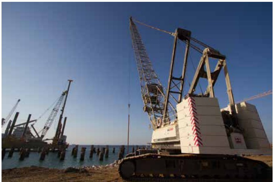
Top and above: Mota-Engil uses the Terex HC 230 and HC 275 crawler cranes to carry out various activities on the project, such as dredging, placing rocks and stakes (pillars supporting the pier being built).
