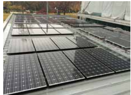
The roof of the store is installed with Panasonic's photovoltaic power generation system.
