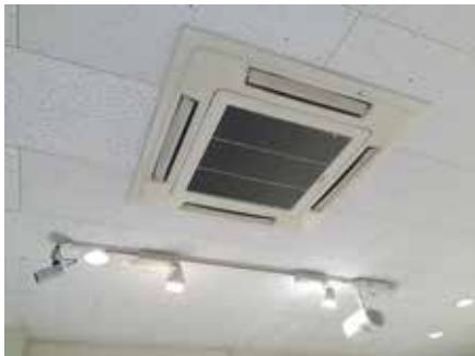
The store is installed with Panasonic's Inverter Split-Type Air-conditioner.
