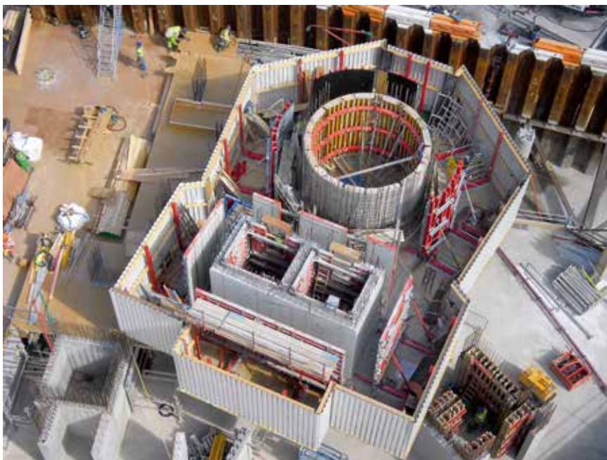
Construction is underway on 866 apartments as part of phase one of the Battersea Power Station development project in central London. Custom-made Rundfix internal circular shutters with the all-plastic facing sheet alkus are being combined with MEVA's new steel formwork system 'Radius' to achieve a class B concrete finish. MEVA's large-format wall system Mammut 350 seen here on the guided climbing system MGC, has a load capacity of 100 kN/m 2 . Its 3.50 panel enables the contractor to finish one level in a single pour from ground to roof using just one panel height.
