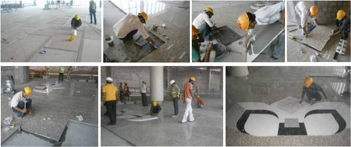
In these photos: Brazilian Santa Cecilia granite, bonded with KERAFLEX MAXI S1 and KERALASTIC T, was used for the flooring in the airport.
