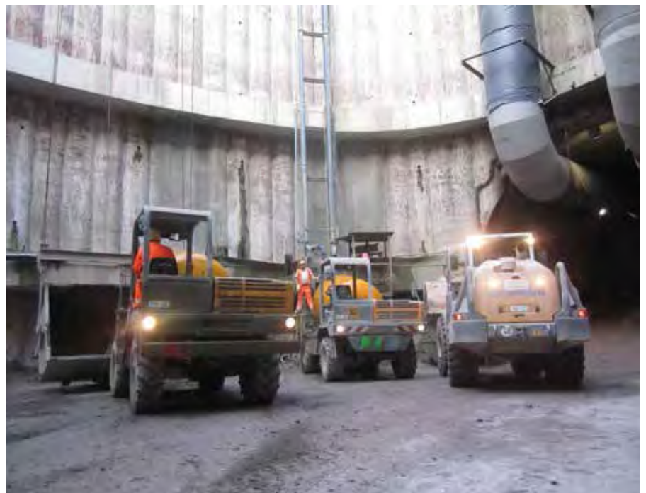
Top and above: Liebherr R 944 C Tunnel crawler excavators are working hand-in-hand with Liebherr L 556 Tunnel wheel loaders in the ARGE 'Tunnel Cannstatt'. Many other items of special tunnelling equipment from Liebherr are also being used in the overall Stuttgart - Ulm rail project.
