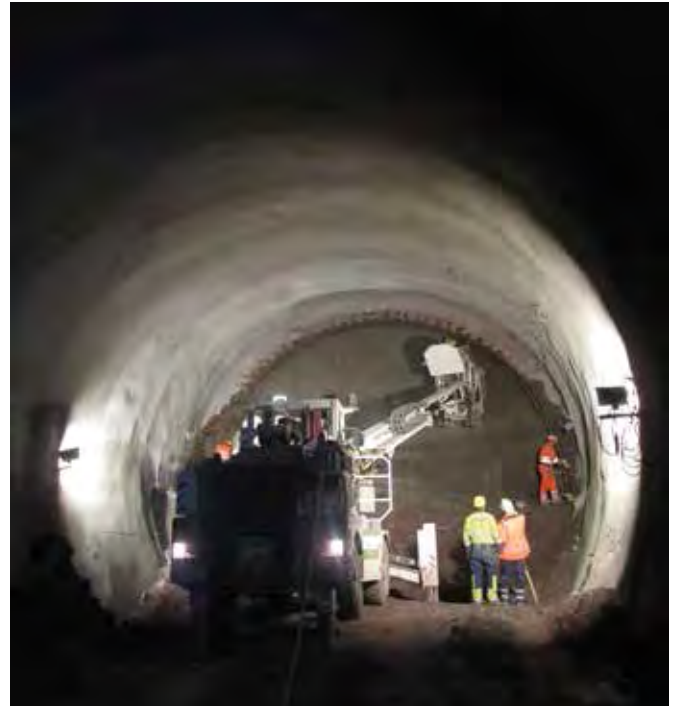
A total of 16 tunnels will be built as part of the Stuttgart 21 project.
