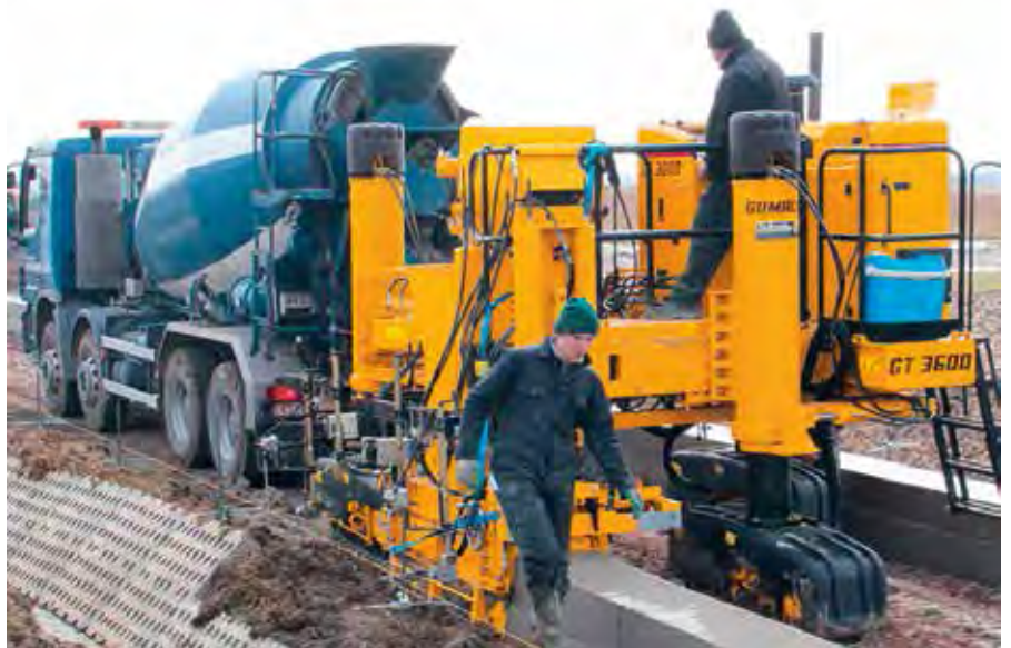
The concrete for the flood retaining wall was a standard Belgian mix design with slump averaging 40 mm. It was delivered to site by ready-mix trucks carrying 9 cu m loads.
