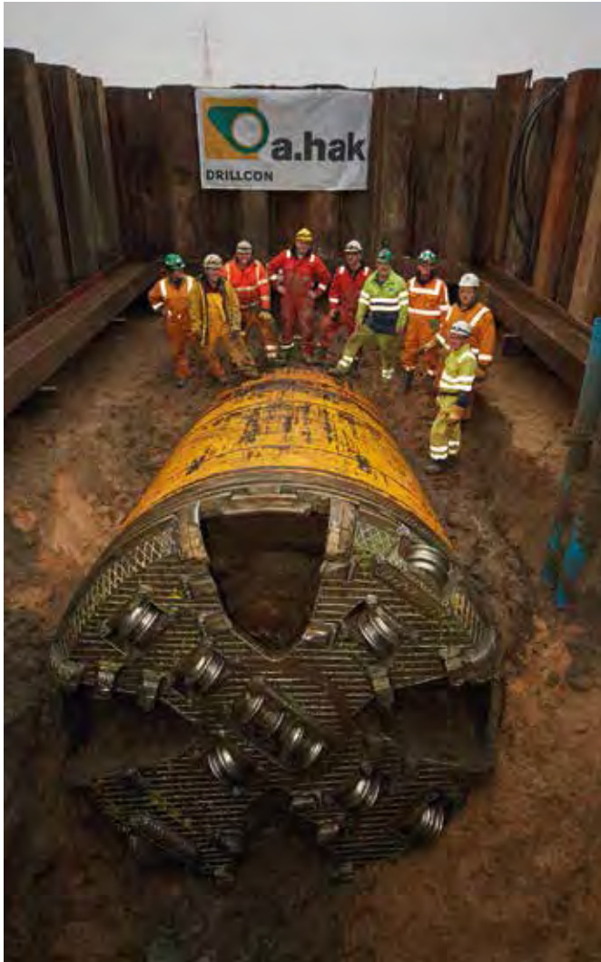
A.Hak Drillcon celebrates the successful breakthrough on Lühensand Island on the Elbe.
