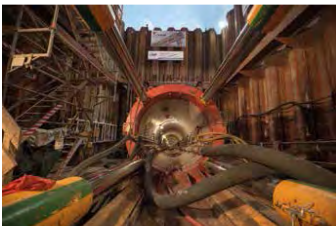
The project team succeeded in steering the AVND2400AB TBM right along the specified route and precisely into the target shaft.
