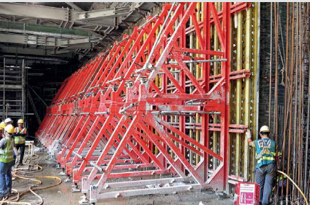
SB brace frame and VARIO GT 24 wall formwork for casting of walls.
