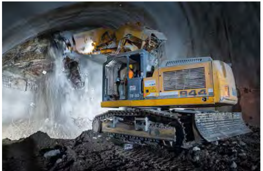
In the Stuttgart 21 project, eight Liebherr R 944 C Tunnel crawler excavators are tunnelling using the shotcrete method.
