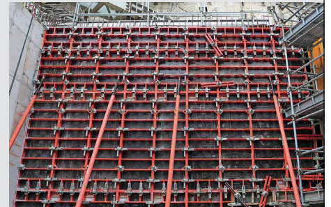
The lightweight DOMINO panel formwork can be assembled with minimum crane assistance.
