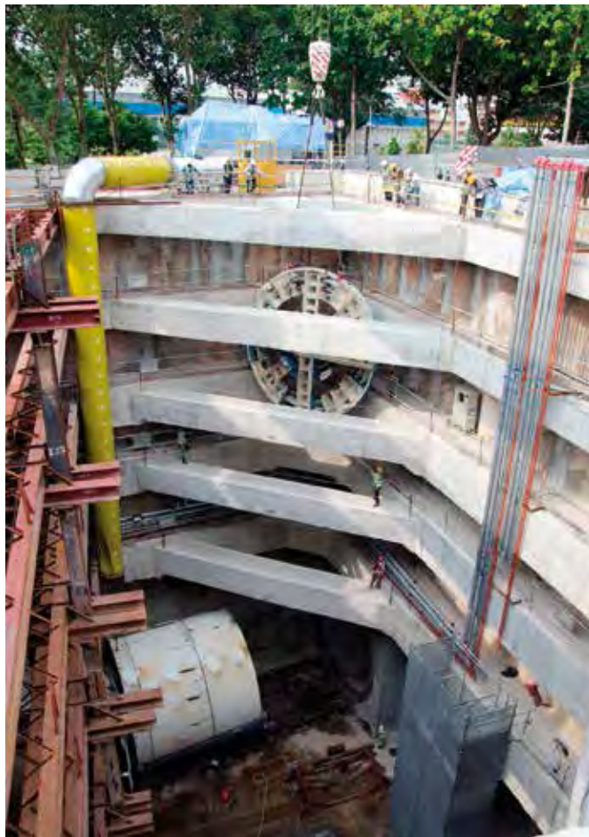
A cutterhead is lowered within a small opening of the shaft at CMC di Ravenna’s C927 jobsite.
