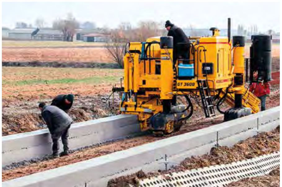
Aannemingen Sico slipformed the retaining wall for flood defense using its new Gomaco GT-3600 curb and gutter machine. The wall is 500 mm wide and 600 mm high.
