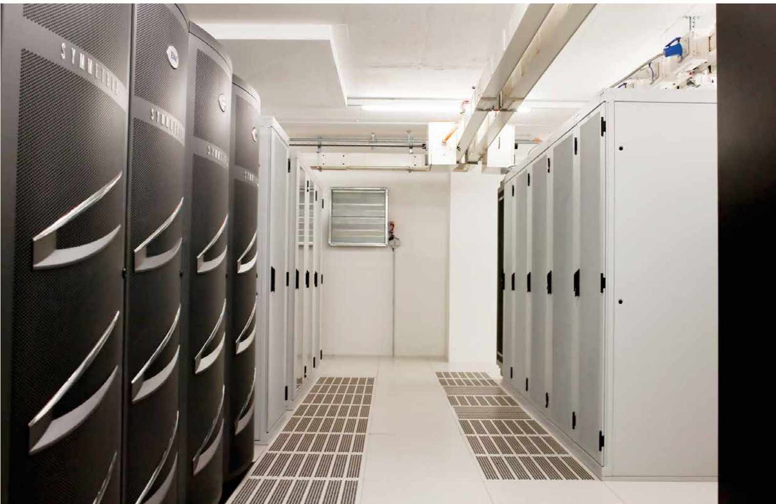
The seamless interaction between fire detection and extinguishing is a basic requirement for ensuring effective fire safety and minimum downtime.
