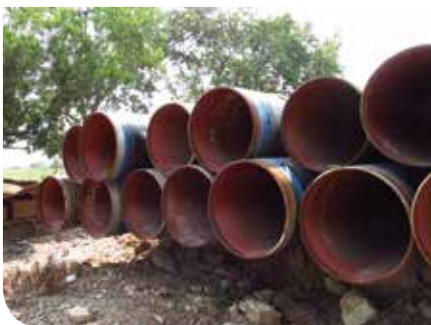
The 28-in pipe will be installed parallel to an existing 30-in pipe, with a separation distance of only 4 m.
