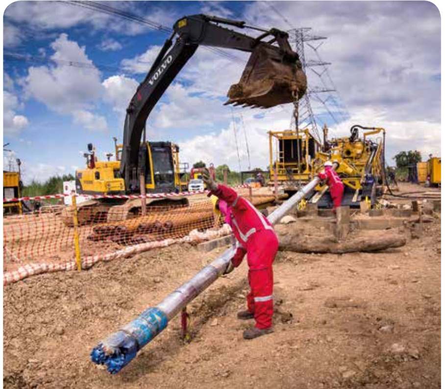
Strega’s HDD team gets ready for pilot bore drilling. The D1000 X 900 rig features a 125,120 Nm rotational torque and a 1,000,000 lbs pullback force.
