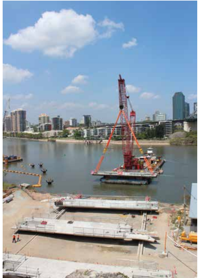
Here, one of the concrete elements is suspended from the SyncHoist’s four yellow hydraulic lifting points controlled by the crane driver, while other concrete elements are slid into position for loading.
