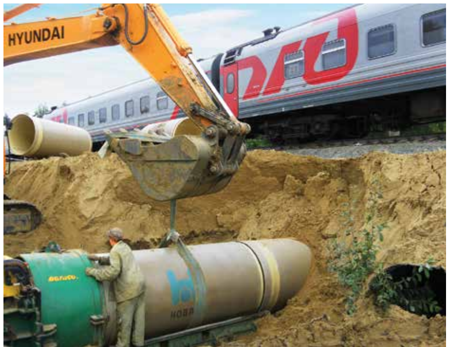
Jacking of HOBAS GRP pipes De 1434 and 1638 beneath a railway section in Russia.
