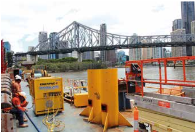
The Enerpac SyncHoist technology was used on the project to handle concrete elements.
