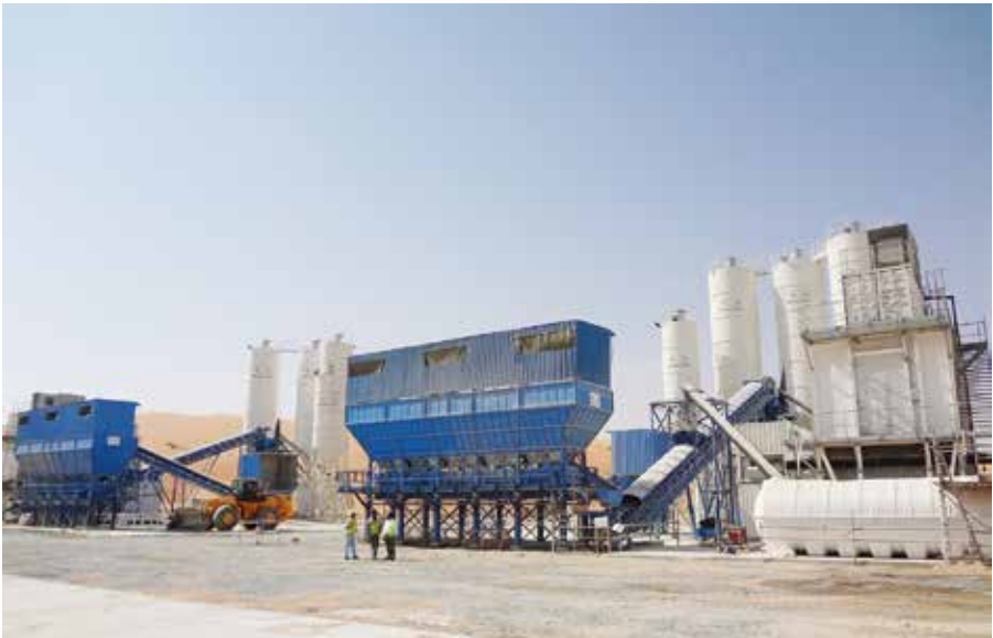
Two Eurotec 5MZ3000T batching plants have been working to supply concrete for the expansion of a refinery in Abu Dhabi.
