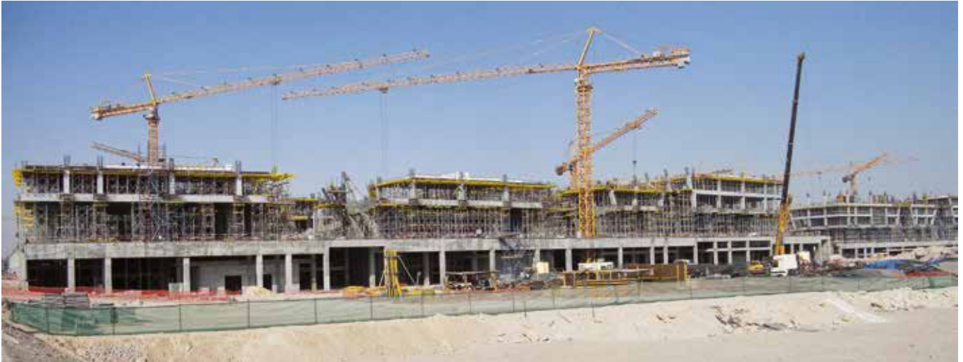
The slabs are being erected by Doka's Staxo 40 load-bearing tower and Dokaflex 1-2-4.
