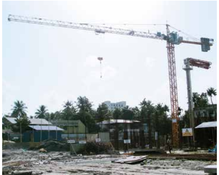
The Potain MCi 85 A belonging to Technoteam Constructions working on the Travancore Opus Highway project. The crane is erected internally and will climb as the building grows to its final 27-storey height.
