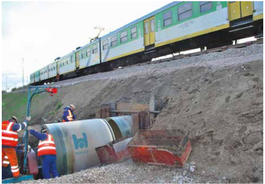
Jacking of HOBAS GRP culverts De 1720 and 2047 under a rail line in Poland.
