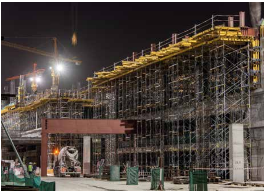
Top: The new Sabah Al Salam University City in Kuwait is currently under construction. Work on the project started in 2013 and is expected to be completed this year.
