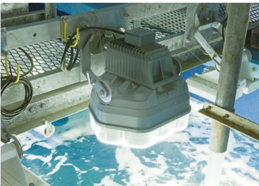
High-output LED floodlights (LEDioc FL400) have been installed in the large Sea of Japan tank, which has a water capacity of 800t
