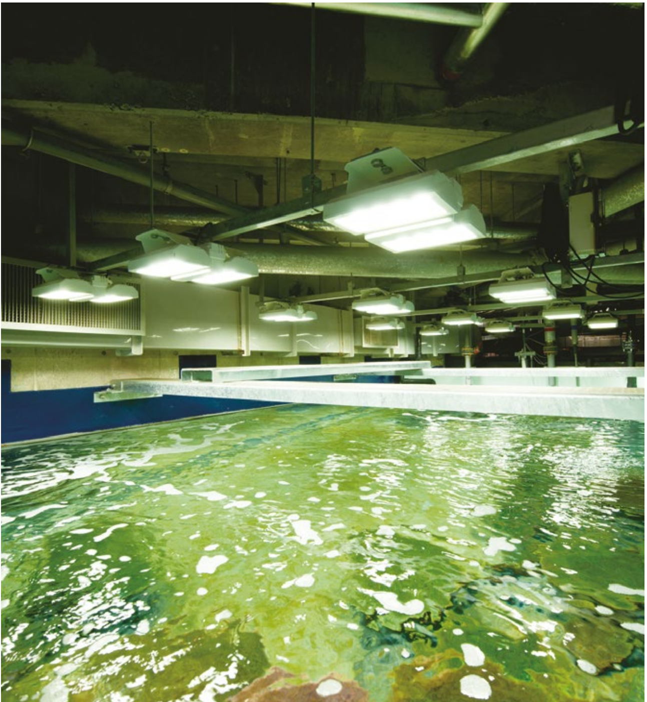
The lighting fixtures installed in the tank top sections are LED high-ceiling lighting fixtures (LEDiOC CEILING HB)
