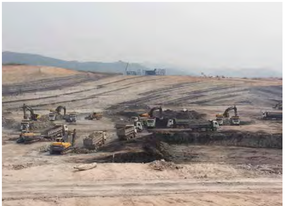
Top: The Hongsa Power Plant in Laos.
