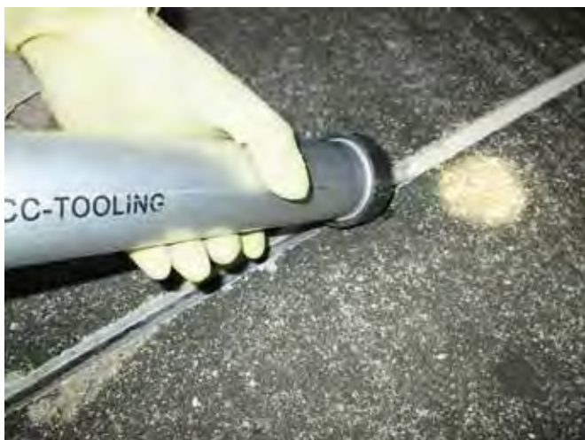
Flexible joints among new concrete slabs were sealed with Mapeflex PU50 SL paintable, castable polyurethane sealant.
