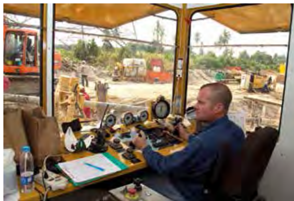
Top: Many onshore gas pipeline projects in Thailand are now being carried out using the HDD method.
