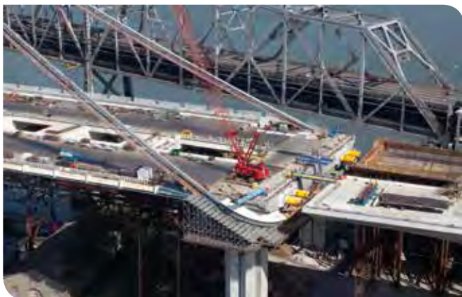
Designed to minimise the weight of the anchorage, the loop at the west bent is the first application of its kind in the world.
