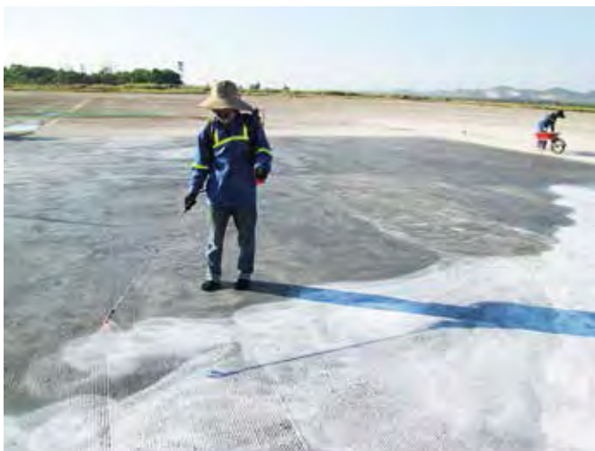
To protect fresh concrete slabs from rapid water evaporation caused by wind or sunlight and reduce surface cracking, Mapecure E anti-evaporation agent in water emulsion was sprayed on the concrete surfaces.
