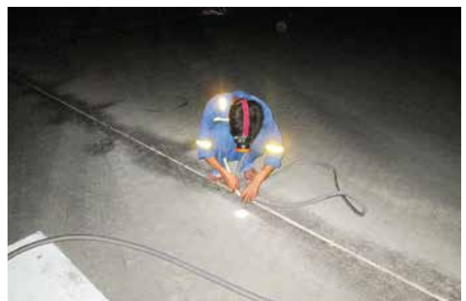
To regulate the depth of Mapeflex PU50 SL, Mapefoam closed-cell expanded polyurethane flexible cord was inserted beforehand in the joints.
