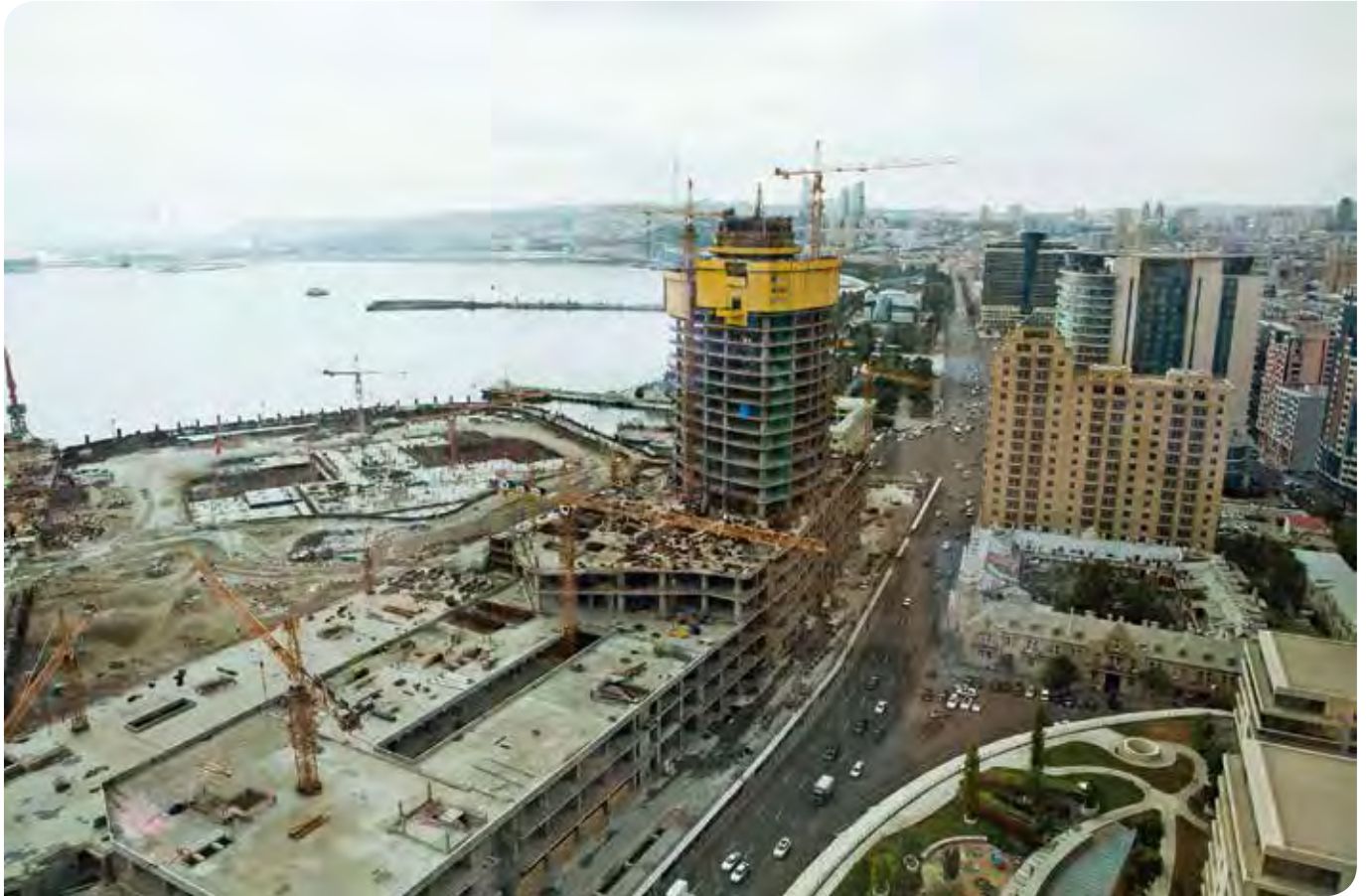
The Doka SKE50 and SKE100 automatic climbing formworks ensure unrestricted construction progress at both high-rise buildings during any wind and weather condition.
