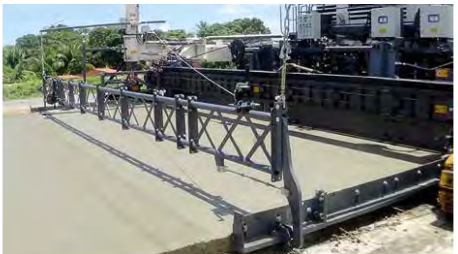
Finishing beam and super smoother ensure an excellent surface when paving large concrete areas. An eccentric moves the finishing beam back and forth perpendicular to the direction of travel, smoothing the surface.
