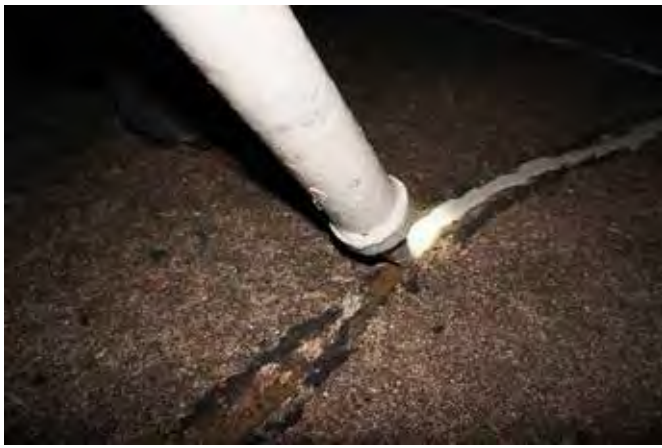
Mapeflex PU50 SL was also used to seal cracks on the surfaces.
