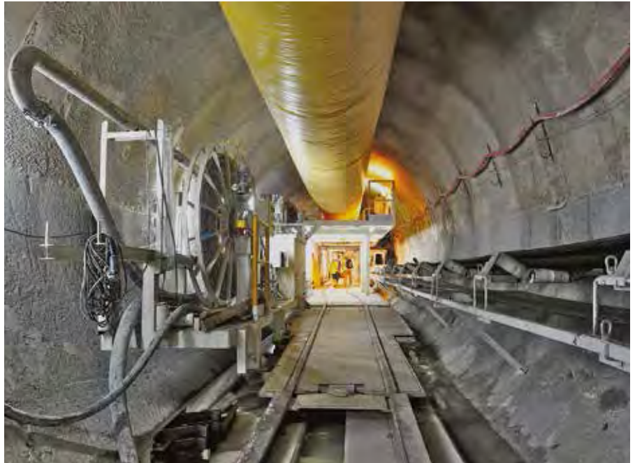
Above: The near-zero rebound system, with its quick set time of 30 minutes, saved a significant amount of time compared to conventional ground support methods.
