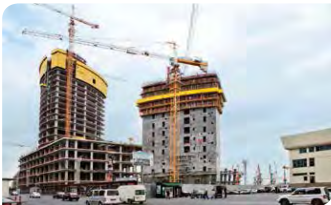
Crescent Place will feature an eight-storey shopping centre with a 170 m high residential tower. Next to it, the 203 m high Crescent City office tower will overlook the entire area.
