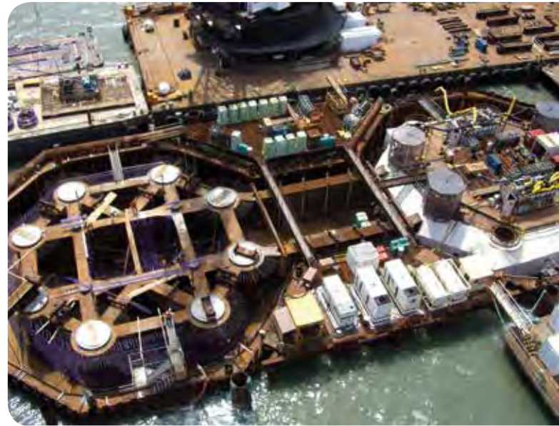
The east bent is supported by 16 2.5-m diameter cast-in-steel-shell concrete piles support. These vertical piles are about 100 m long, among the longest piles ever used for a suspension bridge, and are founded on bedrock.
