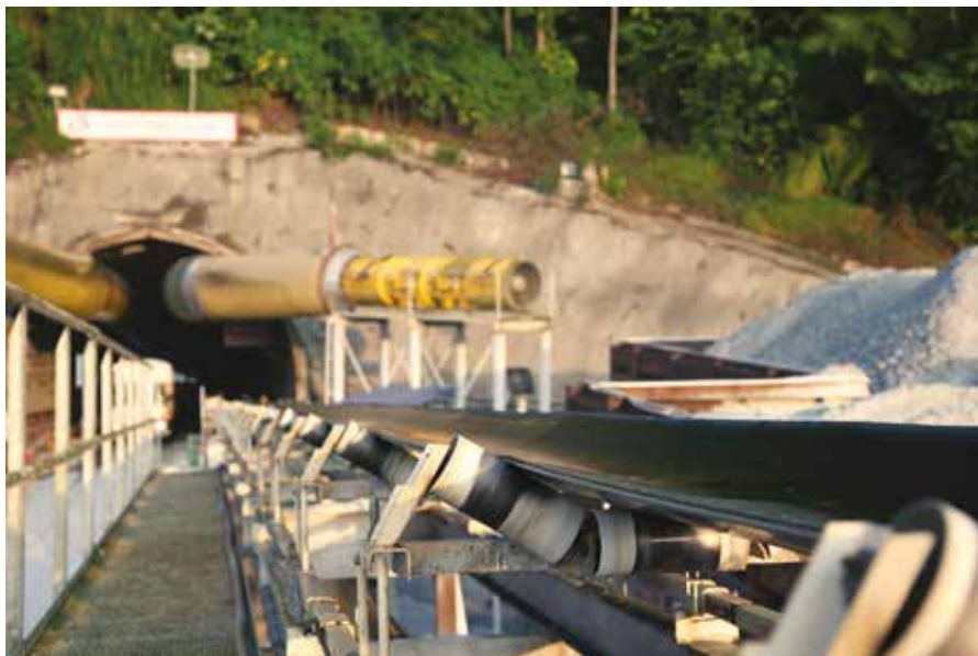
Three Robbins continuous conveyor systems operated simultaneously behind each TBM, averaging 92 percent availability.
