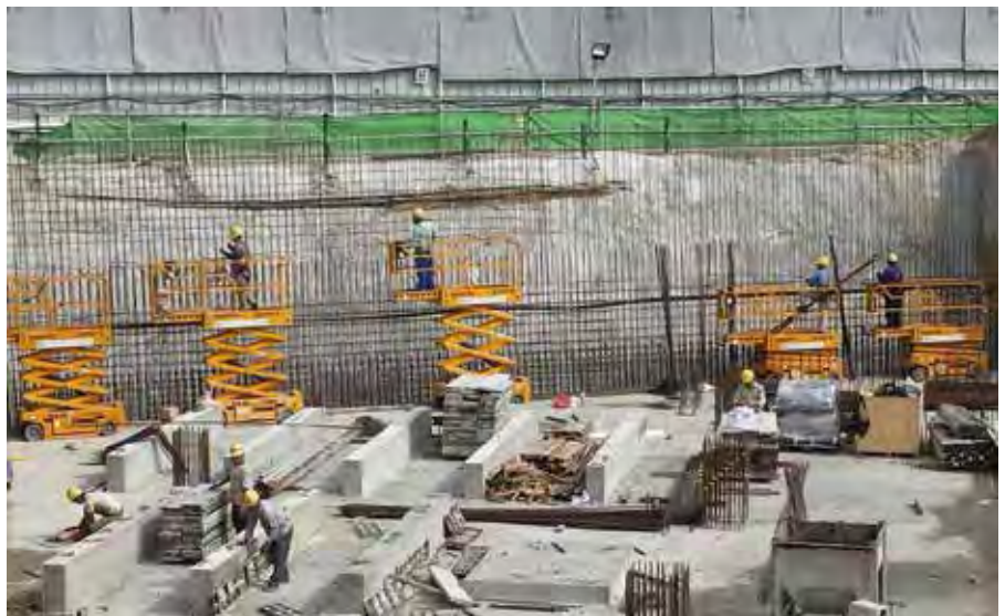
Haulotte Optimum 8 scissor lifts being used at the Bedok Integrated Complex in Singapore, which is built as part of an initiative to revitalise Bedok Town Centre. Designed to be robust, reliable and easy to maintain, the scissor lifts have a working height of 7.8 m and a lifting capacity of 230 kg.
