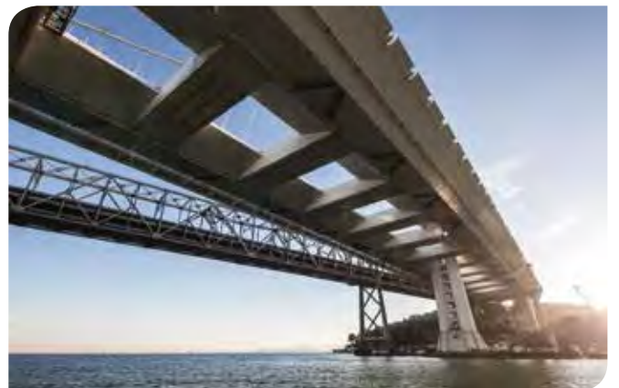
The cross beams also ensure that the dual box girders act composite during wind and seismic loads (Verendeel truss action).
