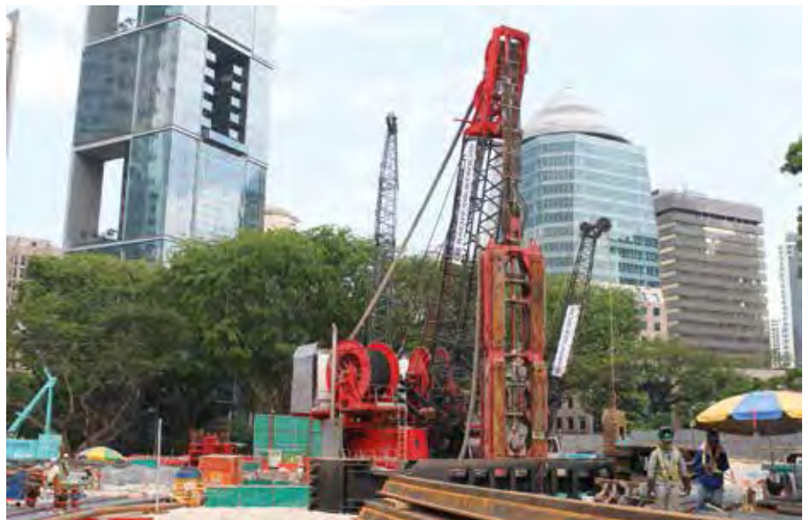
Top and above: A joint venture between Penta-Ocean Construction Co Ltd and Bachy Soletanche Singapore Pte Ltd is currently building the Orchard Station as part of Singapore's Thomson Line project.
