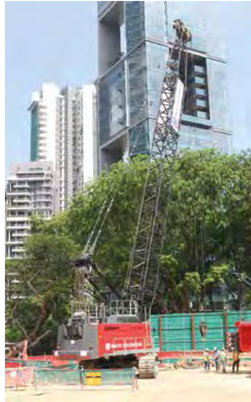
The Liebherr HS 855 HD duty cycle crawler crane being used on the project has a lift capacity of 90 t and is equipped with a hydraulic diaphragm wall grab powered by the crane engine.
