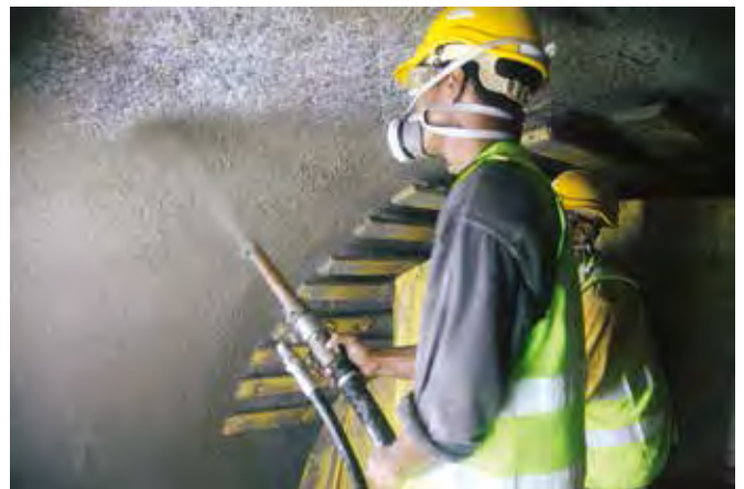
A novel type of polypropylene fibre shotcrete was applied as the primary means of ground support - a mixture that dramatically reduces rebound.
