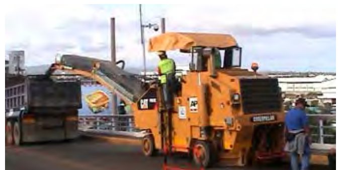
A Cat PM102 cold planer was used to help repair the Mandaue-Mactan Bridge asphalt pavement.
