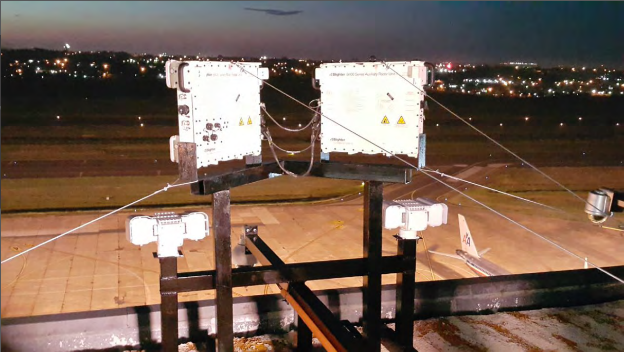
Figure 2 – Typical installation of 180-degree e-scan Doppler radar at a large international airport in South America
