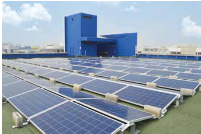
Solar panel systems on the roof of Extra Space Asia's Kallang Way facility.
