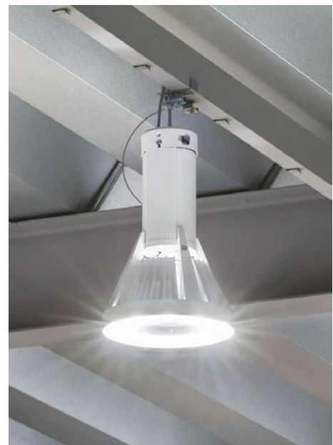
The installed LED high-ceiling lighting fixtures (LEDioc HIGH-BAY \Lambda wide angle light dispersion). The uniform and high-brightness lighting has realized safety and a high-productivity work place environment.
