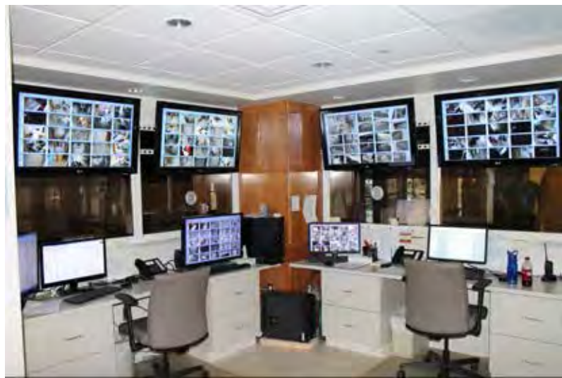
The Security Office at Highland-Clarksburg Hospital allows staff to manage the access control and video surveillance at the facility.
