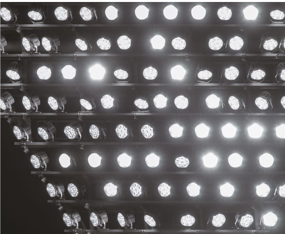
LEDioc FLOOD DUELL LED floodlights with three kinds of light distribution—medium/wide/super-wide-angle—have been installed on the lighting towers.
