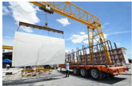
VCON white glass fiber reinforced concrete panel is being shipped to Emquartier. Photo: © VCON Group
