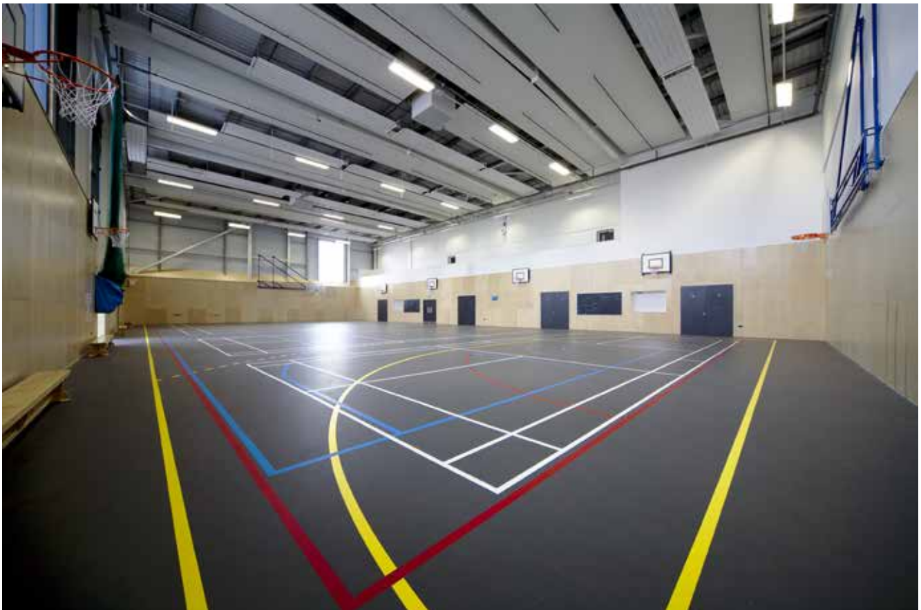
ZIP Radiant Heating Panels installed at Plymouth School of Creative Arts in Devon. Photo: © Zehnder Group UK Limited
