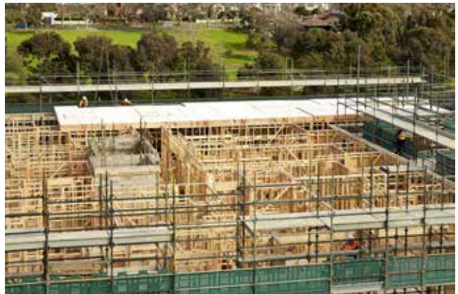
Construction of The Green in Parkville, Melbourne, Australia. Photo supplied by Frasers Property Australia
