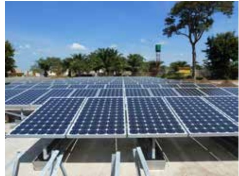
Hybrid Solar / Wind off-grid power plant 110 kW installed in Kashobwe, D.R. Congo.
