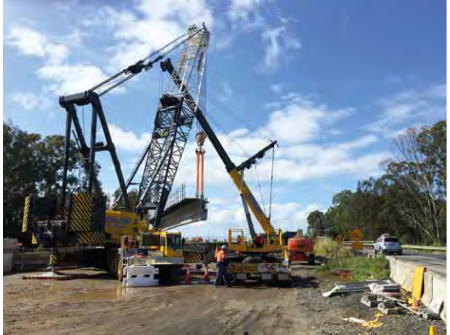
To handle the lifting work on the 117 m long Duck Creek Bridge, Universal Cranes used a 450 t capacity Grove GMK7450 all-terrain crane and a 275 t capacity Manitowoc M-250T lattice boom truck crane. Both units worked in tandem to install 21 bridge beams, each weighing up to 82 t.
