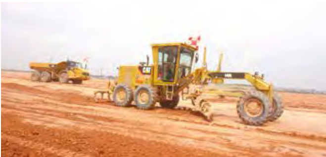
Top and above: Caterpillar's machines carry out land preparation works on the Changi Airport Terminal 5 project in Singapore.
