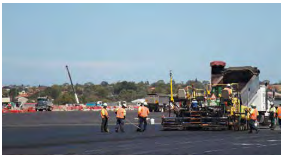
Top, middle and above: The Trimble PCS900 Paving Control System includes a Trimble SPS930 Universal Total Station setup on-site combined with a mast mounted on the tow arm of the paver with a Trimble MT900 prism on top and a slope sensor on the bottom for highly accurate positioning; a radio to communicate with Trimble SPS930 Universal Total Stations; and a Trimble CB460 control box that displays the 3D design model and the position of the screed.
