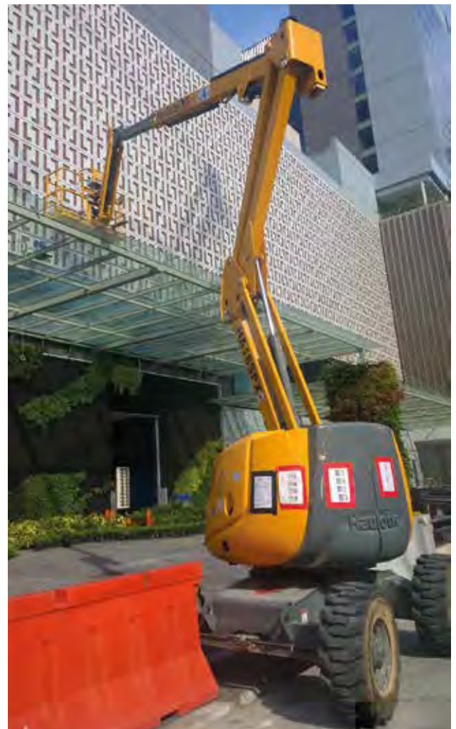
Haulotte HA18 SPX articulating boom lift carries out facade work at Katong Square.
