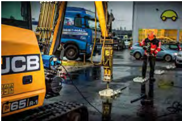
Top and above: Maanrakennus Haapioniemi installs ground anchors with the help of Dynaset hydraulic equipment.
