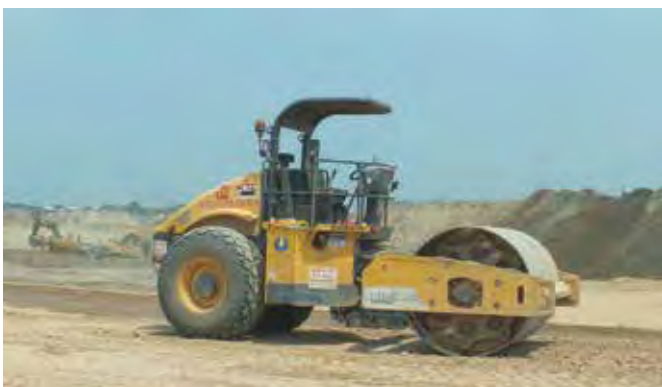
Top and above: A fleet of Volvo machines has been working on Singapore Changi Airport's Terminal 5 project.
