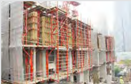
RCS caters for shear walls and lift cores casted ahead of the slab
