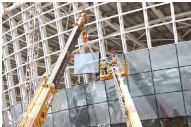
Top and above: Haulotte aerial platforms work on the Abu Dhabi Midfield Terminal Complex– Expansion Project.
