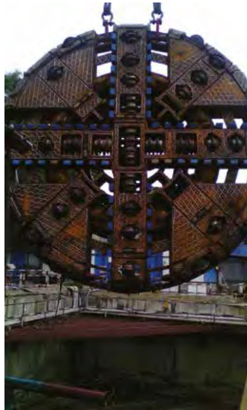
Left: The Robbins EPB bored through unexpectedly hard granite rock in two parallel 1-km drives.
