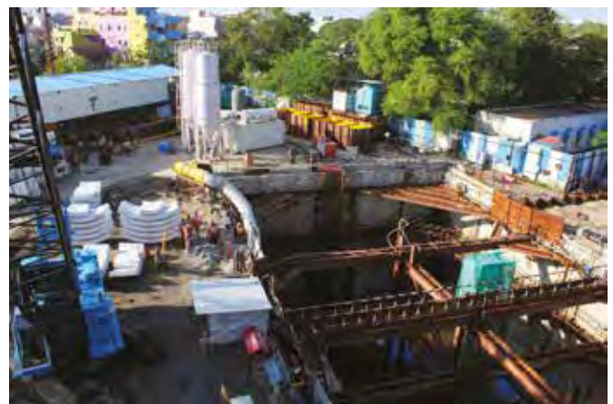
Below: Launched from a 28 m deep starting pit, the EPB experienced challenging ground nearly from the outset.
