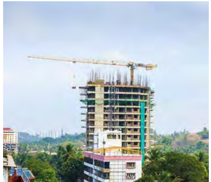
The Potain MCT 85 crane works up to 22 hours a day on the Mangalore Bhandary Heights residential project, lifting concrete, shuttering materials, blocks and structural steel.
