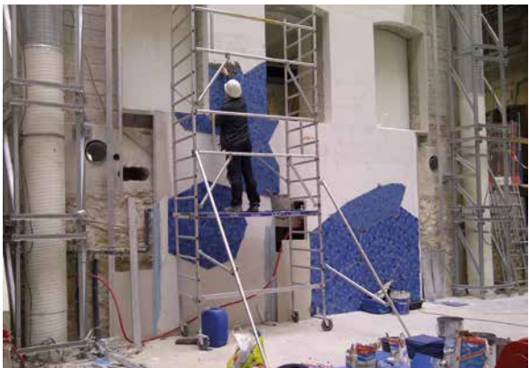
Mosaic was bonded on the floors and some of the walls of Place du Port with KERABOND T+ISOLASTIC.
