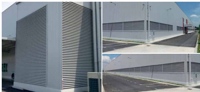
LV3575 Ventilation Louvres from Seng Yoon Seng were used in a distribution centre near the Senai Airport in Johor, Malaysia. Photos: © Seng Yoon Seng
