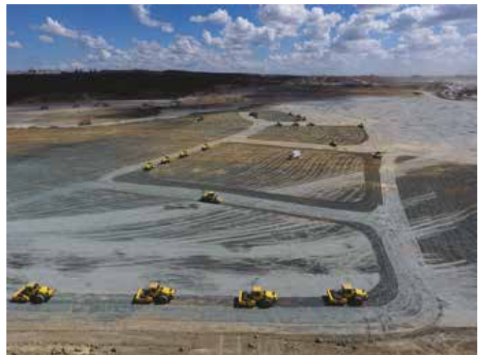
A total of 136 Bomag machines are involved in the project. In five major areas alone, 20 Bomag rollers are working in each zone to compact the surfaces in 40 cm layers.
