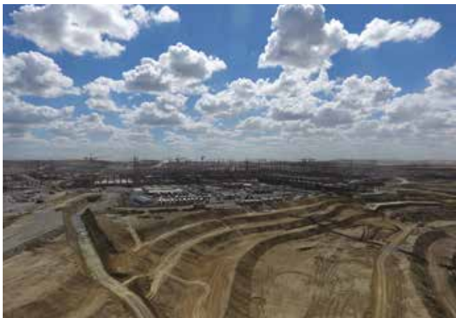
Turkey's new airport is under construction. It is expected to be the world's largest airport upon completion.
