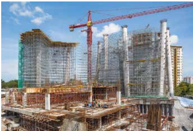
Three elevated high-rise structures for the new SPRM administrative centre. Peri supported the construction progress with an efficient climbing solution, complex shoring construction along with a comprehensive range of services.
