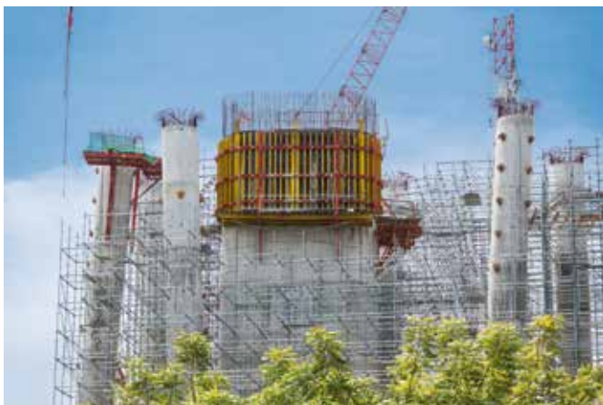
Working scaffold, bracing and shoring all rolled into one: Peri Up subsequently followed as birdcage scaffold within the cycle of the RCS climbing formwork.
