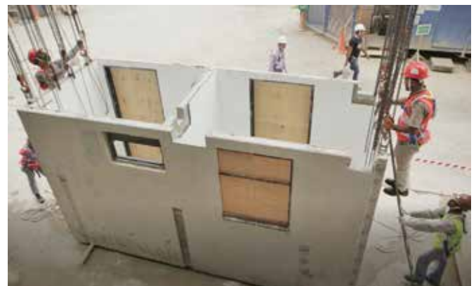
Top (left and right) and above: A new residential development in Singapore is currently under construction, incorporating prefabricated bathroom units (PBUs).
