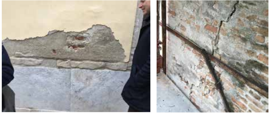
Masonry walls featured damaged and uneven renders.
