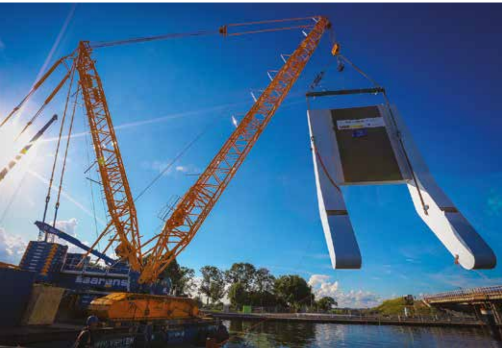
Left: During the bridge's construction, Sarens was tasked by Hollandia Infra to lift and position the two main balanced tail bridge segments weighing in excess of 280 t from barges on the Old Rhine River. The company used a Demag CC 3800-1 crawler crane to complete the job.
