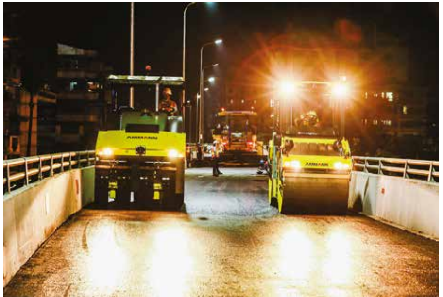
Above and bottom: Various Ammann machines were involved in the construction of a new flyover in Yangon, Myanmar.
