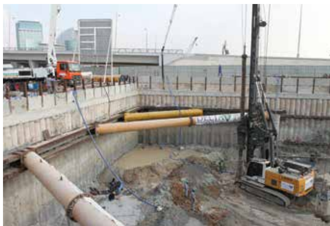
Left: Delta Foundations deploys its Liebherr LB 20 rig to drill 200 piles for a four-star hotel at Dubai's Culture Village development.
