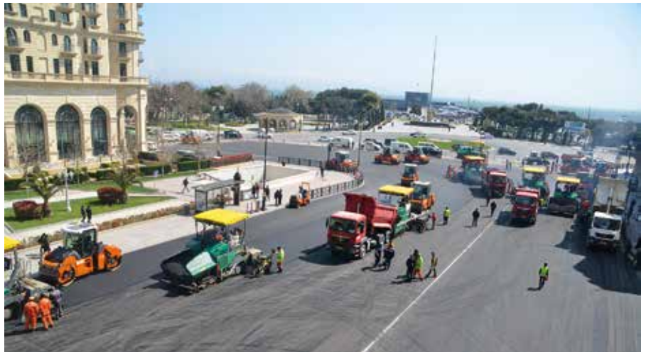
Above: Hot-to-hot installation with Super 1900-2 pavers from Vögele, followed by Hamm rollers.
