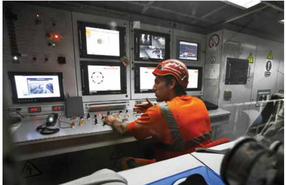
The tunnel excavation was carried out using a TBM named Victoria. The machine is 114 m long and weighs 1,800 t, with a 10 m diameter. It has a rotating head that allows tunnels to be bored and then lined with segmented concrete rings, completely automatically, through both hard rocks and softer ground, or below aquifers.
