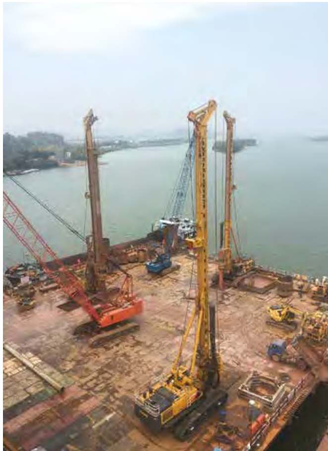
Left: XCMG's XR550 rotary drilling rig at the construction of Xi Jiang railway bridge in Guangzhou, China.
