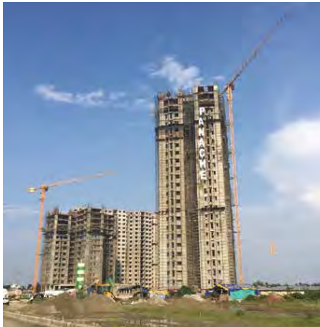
Left: Potain MCT 85 topless cranes work on the PS Panache residential project in India.
