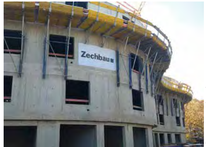
Doka K folding platform keeps the site crew safe all the time.
