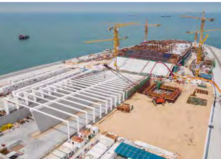
Top: On two artificial islands at both exits of the HKZMB tunnel, striking architectural concrete structures are currently being built. On the right of the picture, the exit at the west end of the tunnel can be seen.
