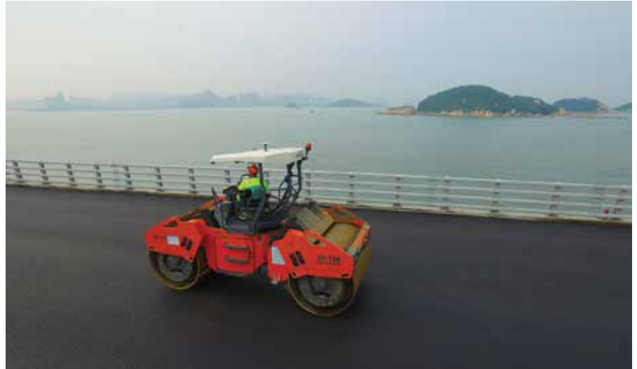
Hamm oscillation rollers at work on the Hong Kong-Zhuhai-Macao Bridge project in China. The oscillation technology allows dynamic compaction to be used on bridges without difficulty.
