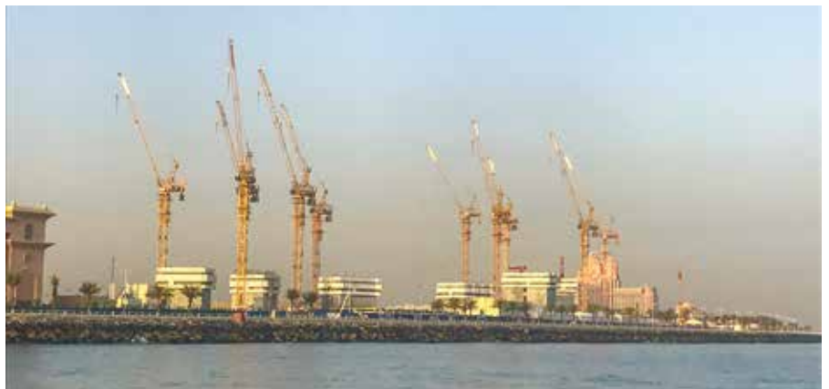
Below: Potain MR 418 tower cranes help build the Royal Atlantis Resort and Residences in Dubai.
