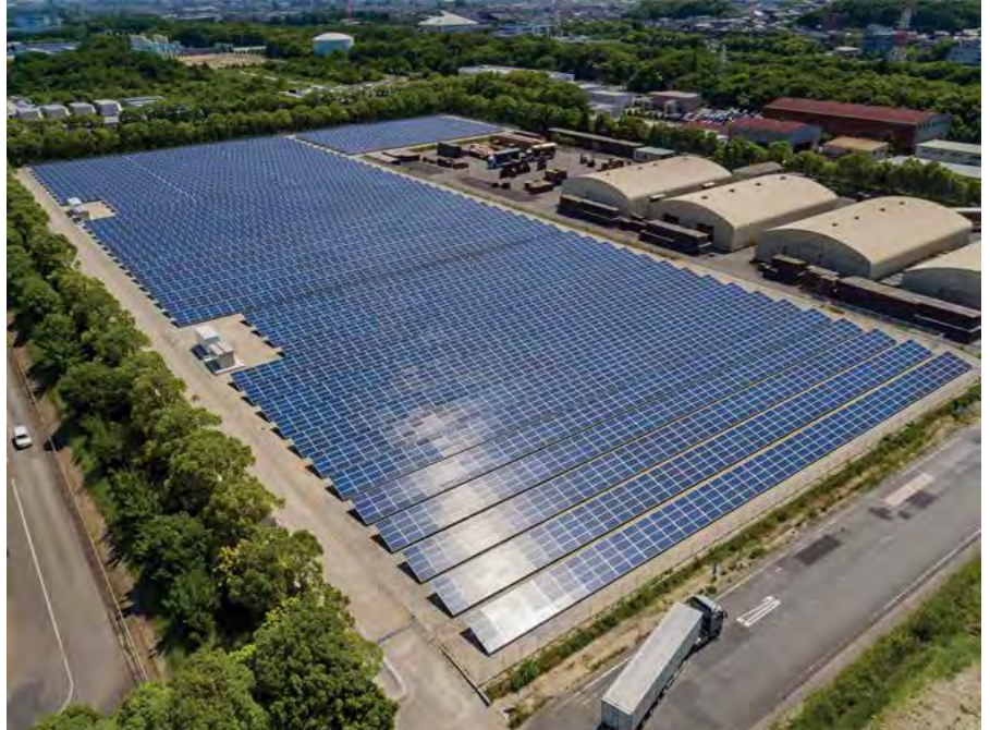
The new Lixil Chita solar power plant covers an area of 52,330 sq m and is expected to offset about 3,000 t of CO 2 emissions each year of operation.
