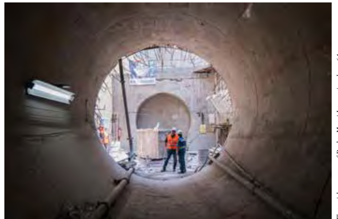
BOTH IMAGES: The new 7.9-km-long Canal General drainage tunnel in Mexico is designed to prevent flooding in the Valle de Chalco area, as well as in the metropolitan area of Mexico City.
