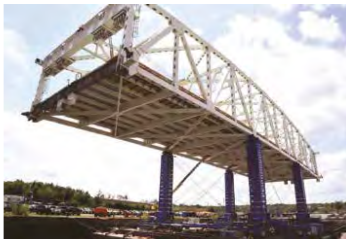
LEFT: The JS500 Jack-Up system being applied in a bridge lifting project. Typical JS set ups employ four 500-t incremental lifting towers, each with a maximum tower height of up to 10 m.
