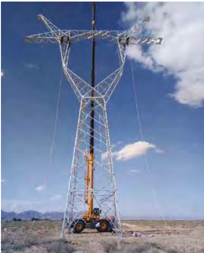
XCMG RT 60 rough-terrain crane installs a power transmission grid in the Alxa Desert.
