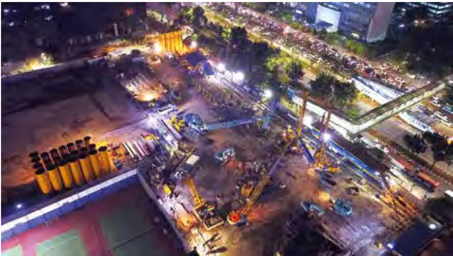
Bauer machines carry out the foundation work for a new 59-storey high-rise in Jakarta, Indonesia.
