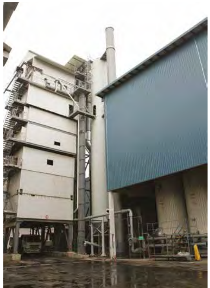
Ammann ABP Universal asphalt mixing plant also helps United E & P to meet strict sound and emissions requirements in a key area of Singapore.
