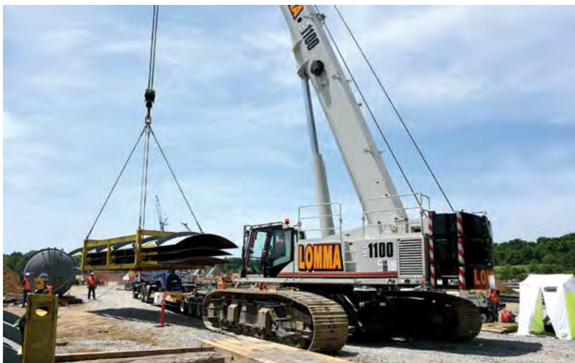
TOP AND LEFT: Link-Belt TCC-1400 and TCC-1100 telescopic crawler cranes being used on the CPV Valley Energy Centre project to unload, sort, and assemble the piping shells at various locations.
