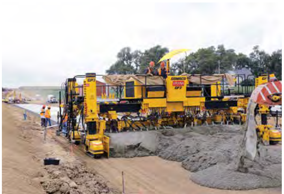
TOP AND ABOVE: Charles Vrana and Son Construction works on a new commercial development in Sarpy County, Omaha, slipforming a new roadway as well as the entrance into the development. The company deploys its Gomaco GP3 paver with a 5400 series mould and bar inserter.
