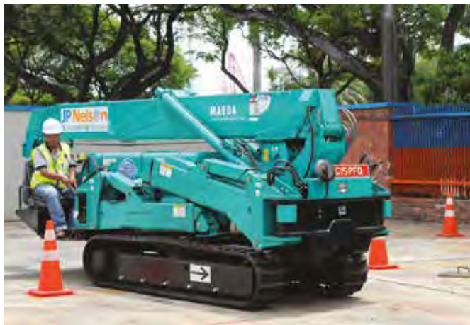
TOP AND ABOVE: The Maeda MC-405C is one of JP Nelson's popular mini cranes in Singapore market. The machine has a compact dimension and can be folded up to enable it fit through a standard doorway.
