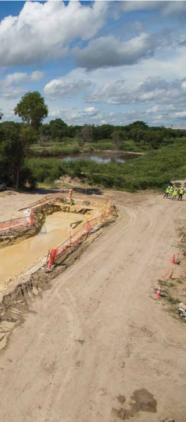
BOTH IMAGES: A new 10-km gas pipeline was under construction in Map Ta Phut, Rayong province, Thailand. HDD contractor Thaitan Drilling Company Limited worked on a 3.5 km section, installing a 28-in-diameter steel pipeline at a depth of 12 m.
