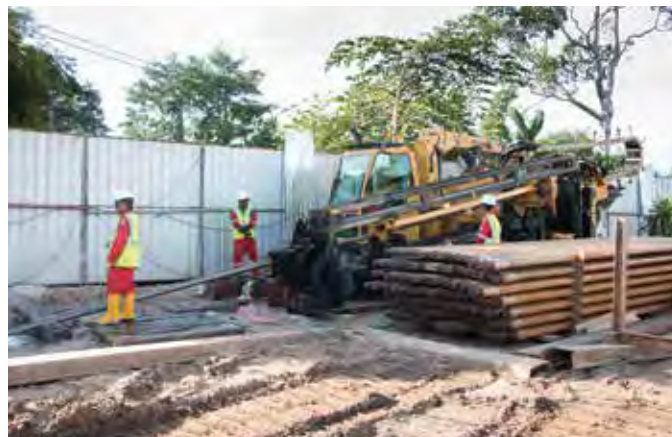
LEFT AND BELOW: The Vermeer D130x150S drilling rig was also working on the project. The machine features 59,000 kg of pullback force and 20,337 Nm of torque.
