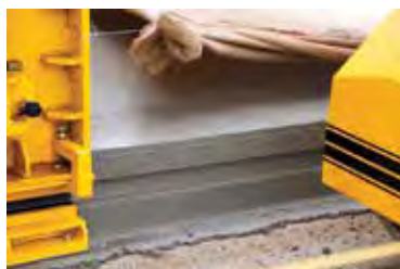
LEFT: The GP3 with 5400 series mould produces a smooth, clean and sharp edge and keyway on this new roadway project.
