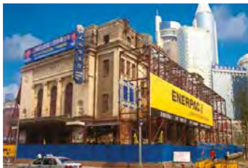
LEFT: The high tonnage cylinders can be used in various industries. Here, they are being used to lift and shift the Shanghai Opera House.
