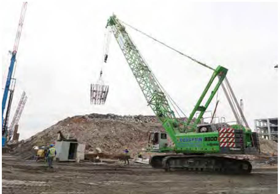
Sennebogen 3300 E crawler crane performs lifting duties on a jobsite at the port of Istanbul, Turkey. The machine's powerful winch rated at 160 kN and rope speed of up to 105 m/min help enable the work to be carried out quickly.
