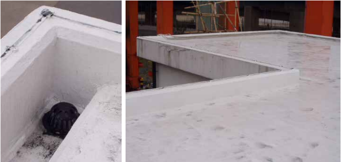
Re-roofing on T8E terminals substations in Hong Kong, done with a similar waterproofing coating system supplied by Eastern Win.
