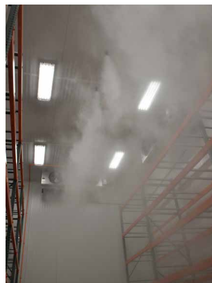
With the introduction of the industry’s first hybrid, water and inert gas fire suppression system in 2009, the industry has responded by developing an applicable standard for this technology; the NFPA is working toward the creation of a new code for hybrid systems – the NFPA 770 Standard on Hybrid (Water and Inert Gas) Fire Extinguishing Systems.
