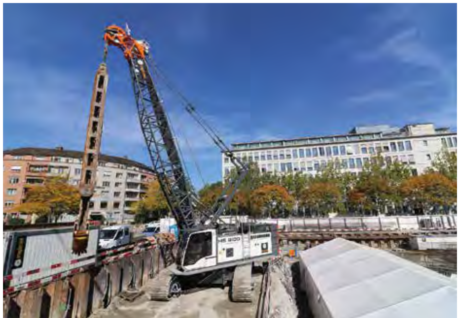
Liebherr HS 8100 HD duty cycle crawler crane works on the redevelopment of Zurich Insurance Group Ltd's headquarters on the Mythenquai, Switzerland.
