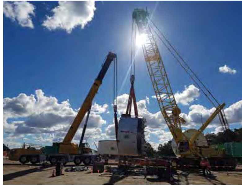
ABOVE: Tutt Bryant Heavy Lift & Shift operates its Manitowoc MLC650 crawler crane to build one of the TBMs, which will be used in the construction of the underground rail system.
