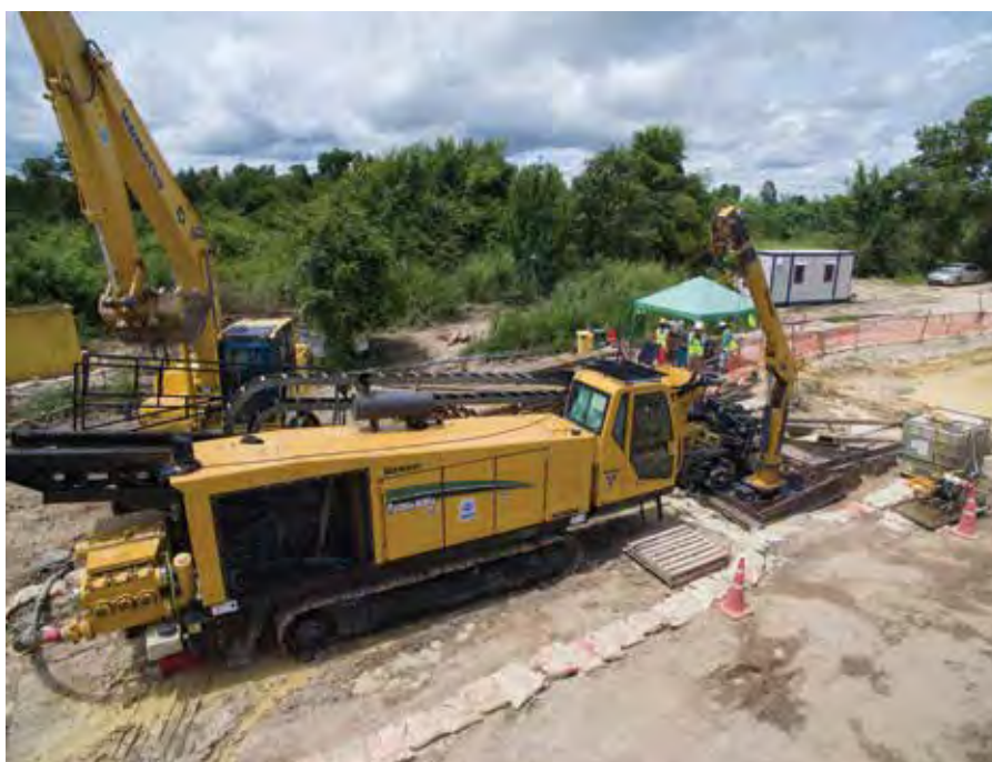
TOP AND ABOVE: The Vermeer D220x300S drill rig is seen here working on a Thailand project. The machine delivers a maximum thrust/pullback force of 100 t, making it suitable for various ground conditions and settings. With a small footprint, it can also operate in congested areas.
