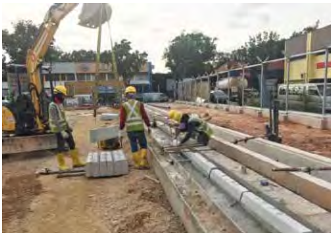
The conventional slipforming method would have taken a longer time, as shown in this image.
