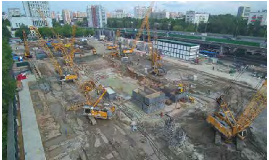
The deep foundation work for a new bus terminal in Moscow, Russia, is being carried out with the help of eight Liebherr machines. These include seven duty cycle crawler cranes and one LRB 255 piling and drilling rig.
