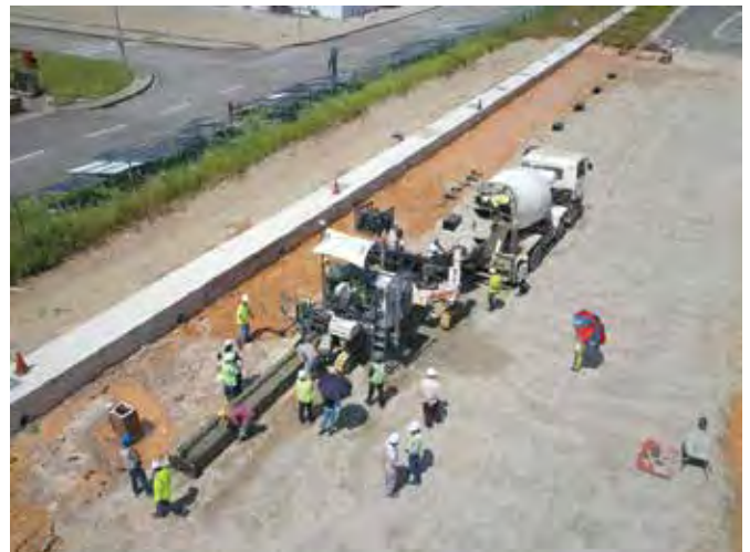
ABOVE: The Wirtgen SP15 slipform paver was chosen for the trial. The machine is equipped with an Autopilot system, thus it does not require any stringline set up and formwork of traditional methods. This saves time and avoids overloading of the surveying team in the process.
