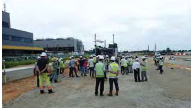
Wirtgen Singapore worked with main contractor Quek and Quek Civil Engineering Pte Ltd to carry out a road paving trial in Tuas South, Singapore.
