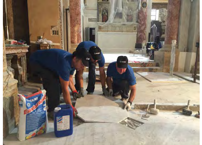
The flooring, made up of slabs of Carrara marble and Bardiglio inserts, was installed using ELASTORAPID two-component cementitious adhesive.
