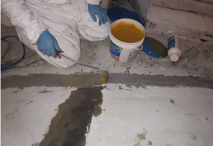
Static structural strengthening work on the dome over the presbytery using the MAPEWRAP system.
